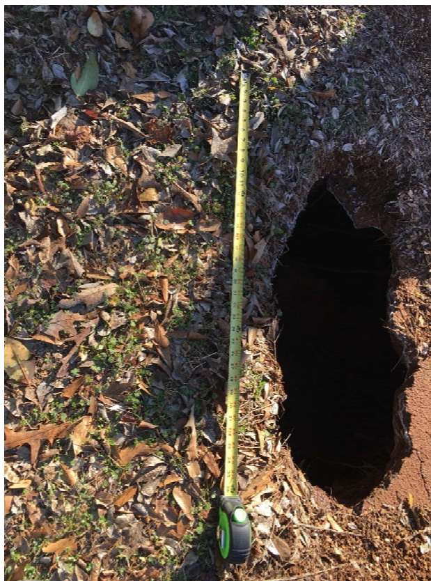
Photo 1: Park St. Sink hole created during the storm.
