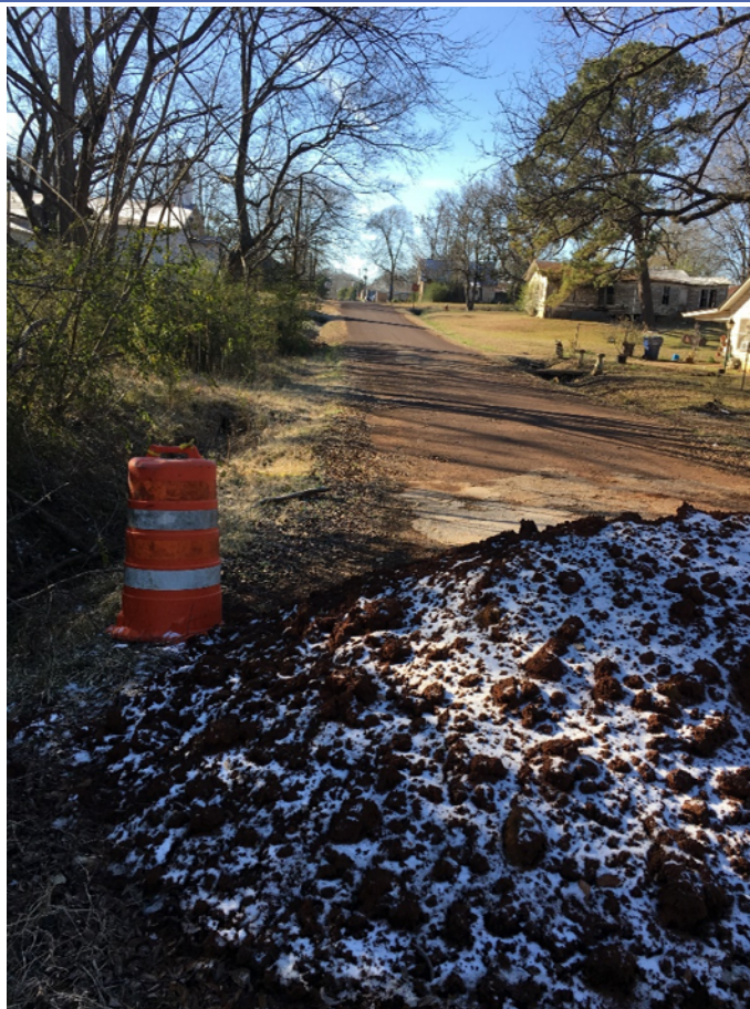
Photo 10: Goldenway looking south. The dirt was placed on the roadway by the city to stop traffic from crossing the bridge/culvert
