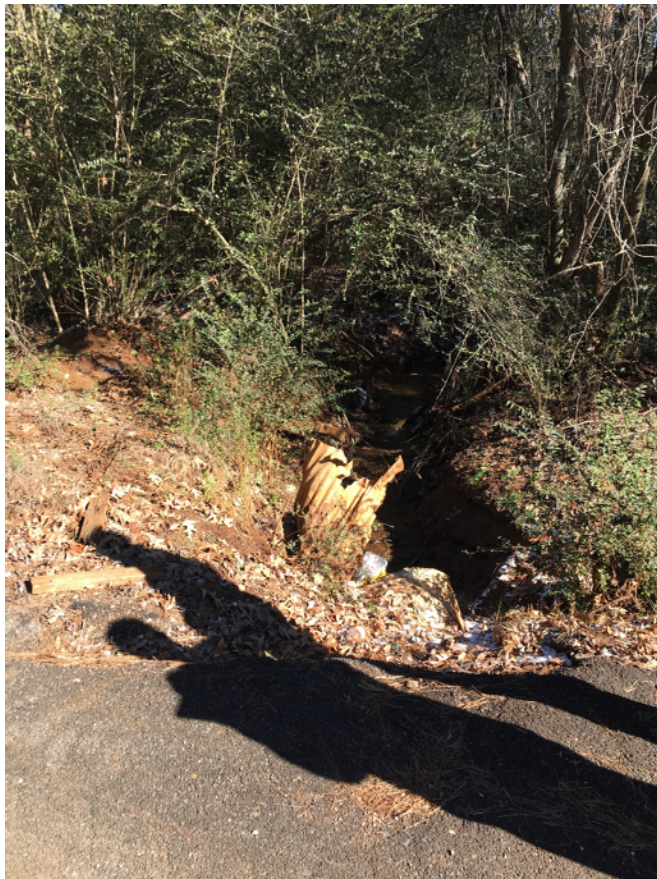
Photo 11: Damaged Culvert on the north side of Bierhalter Rd.
