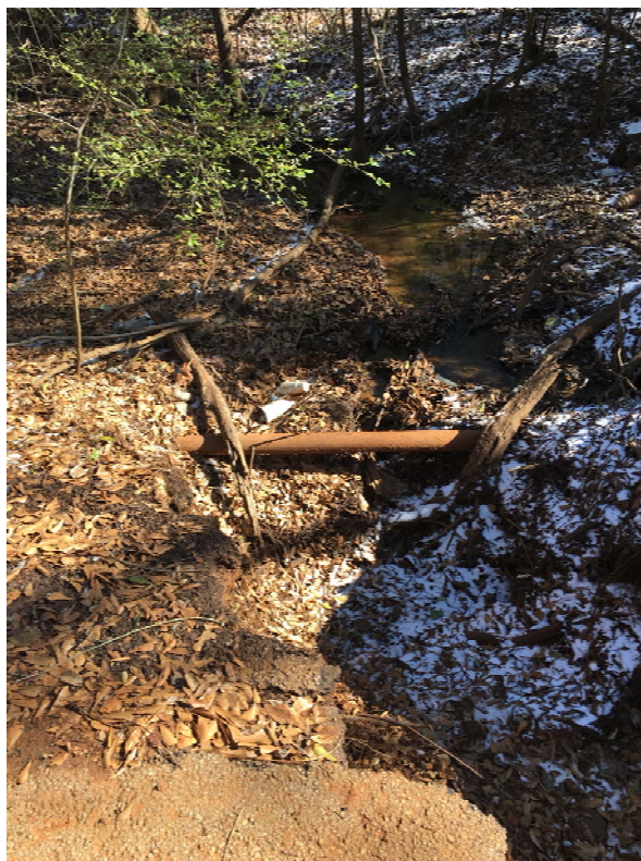
Photo 17: Damage site looking south downstream.
