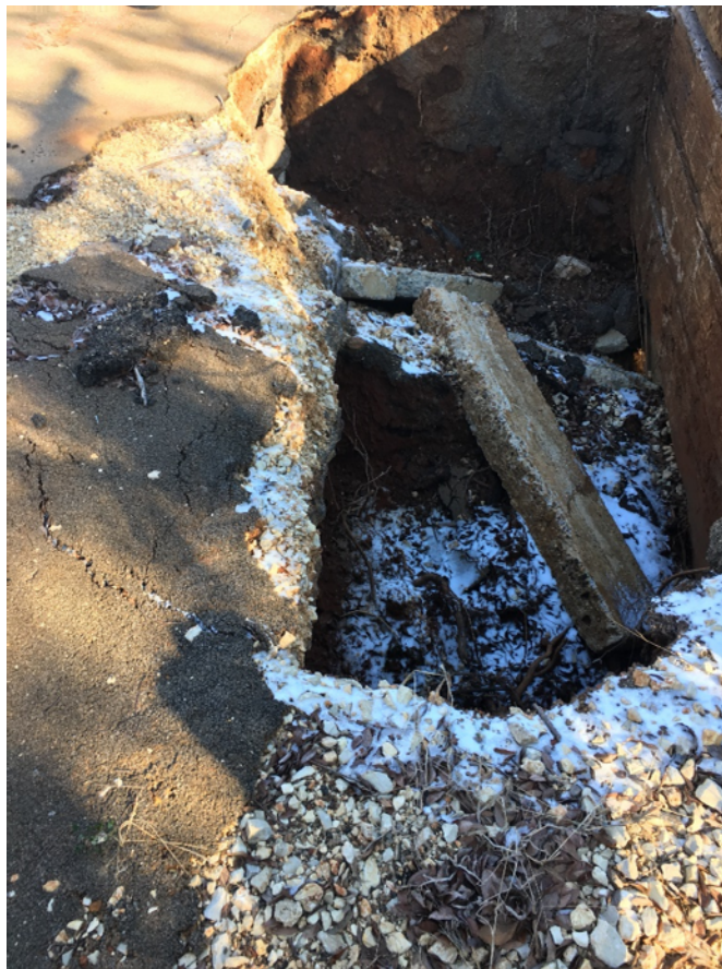
Photo 7: Goldenway Bridge /Culvert showing the degree of erosion that occurred during the storm event.
