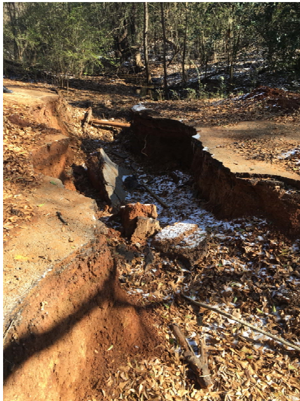
Photo 16: Washout on Milan St. facing west
