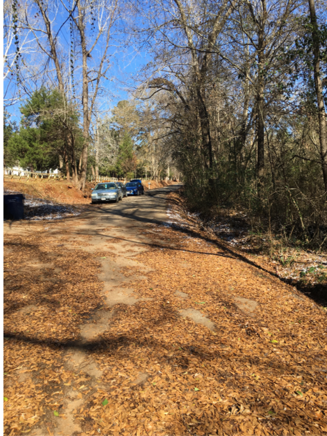
Photo 20: Milan St. looking south from the damaged culvert
