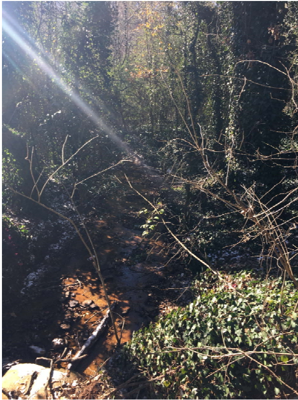
Photo 18: Looking north upstream from damaged culvert (Milan St.)
