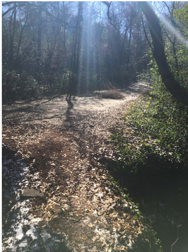
Photo 19: Milan St looking north from the damaged culvert
