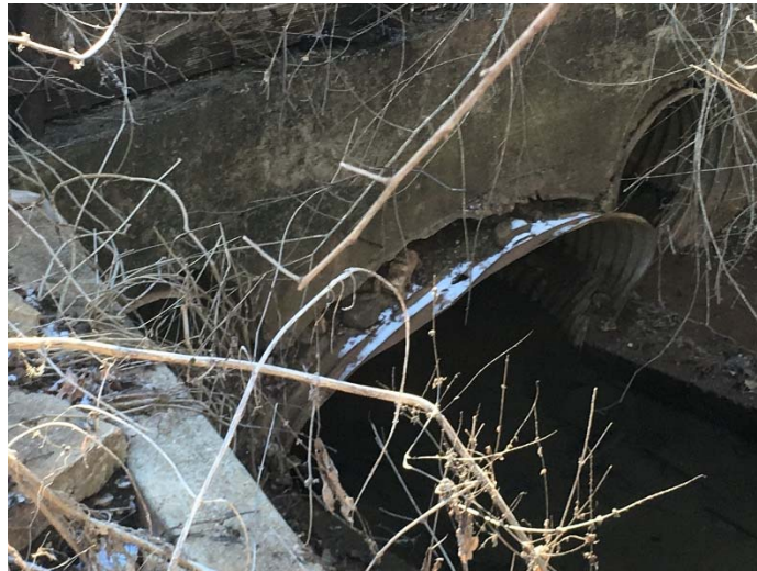
Photo 9: Downstream (west) side of the drainage structure showing main pipe and the overflow pipe
